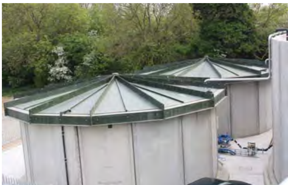
Raw leachate tanks, known as Bletchley and Calvert
