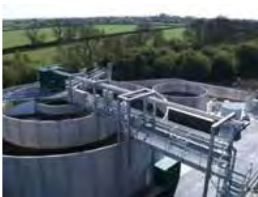
The finished plant where we can appreciate the concentric shape of the LTP
